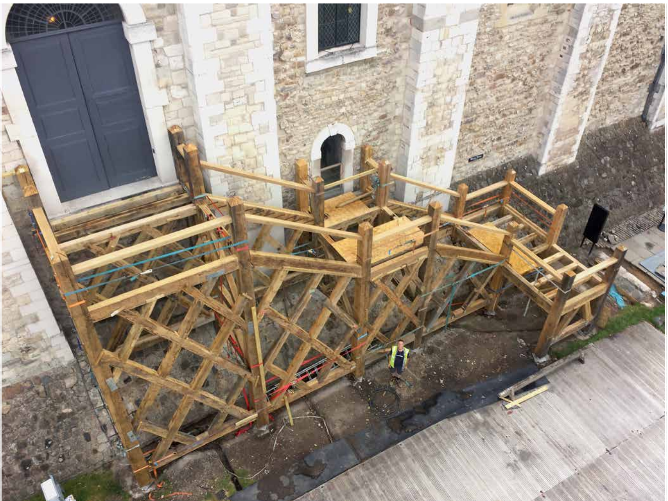
A crane's eye view after most of the principal raising had been completed.
